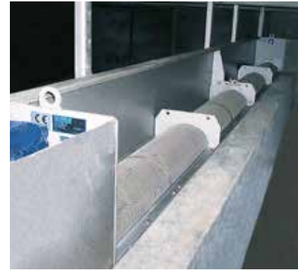
HUBER Storm Screen ROTAMAT® RoK2 installed on foul side of overflow weir.
