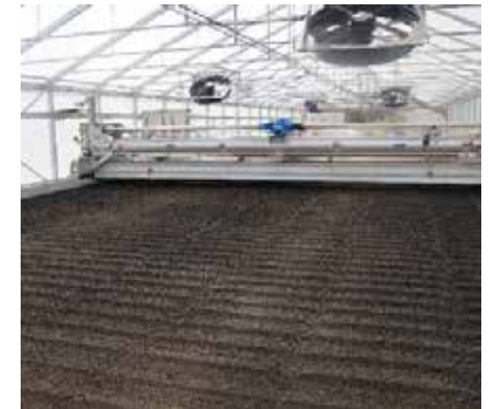
Dewatered sewage sludge becomes dry, stable sludge granulate.
