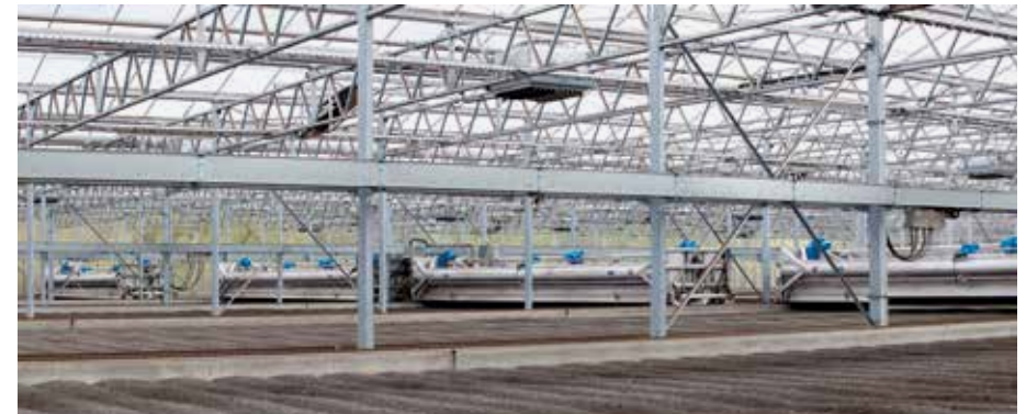
Parallel operation of HUBER Sludge Turner SOLSTICE® units.
