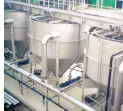
A pair of HUBER Circular Grit Trap HRSF systems.
