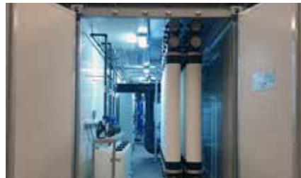
Pre-treatment stage using ultra filtration for suspensions removal.
