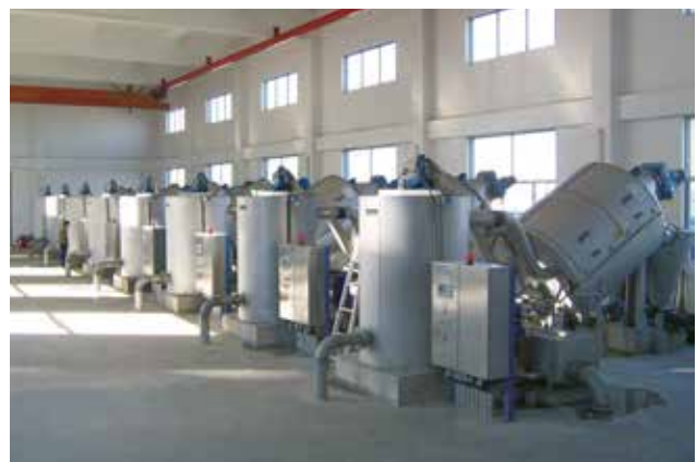
Eight screw thickeners handling 600 m 3 /h.
